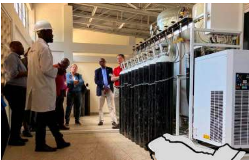
The oxygen plant at Maua Methodist Hospital.
